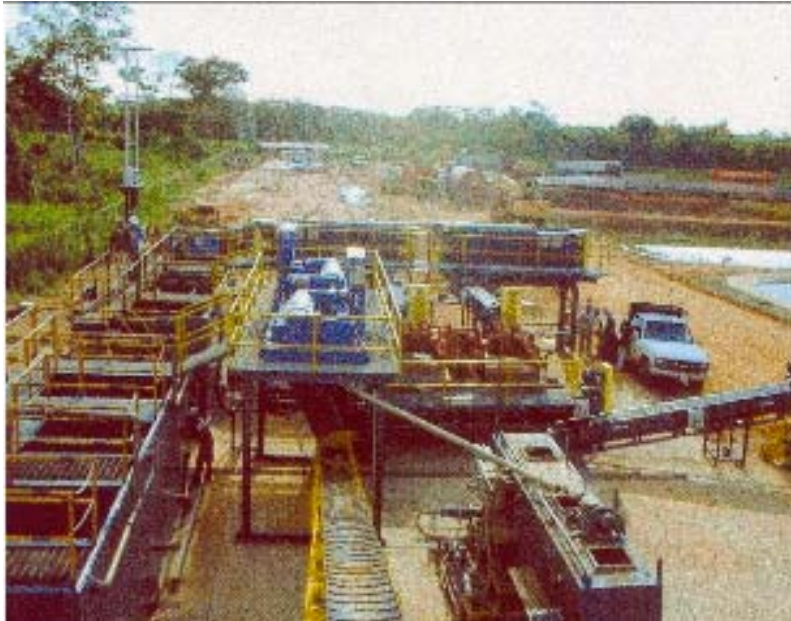
Fig. 1 . Treatment plant on site
